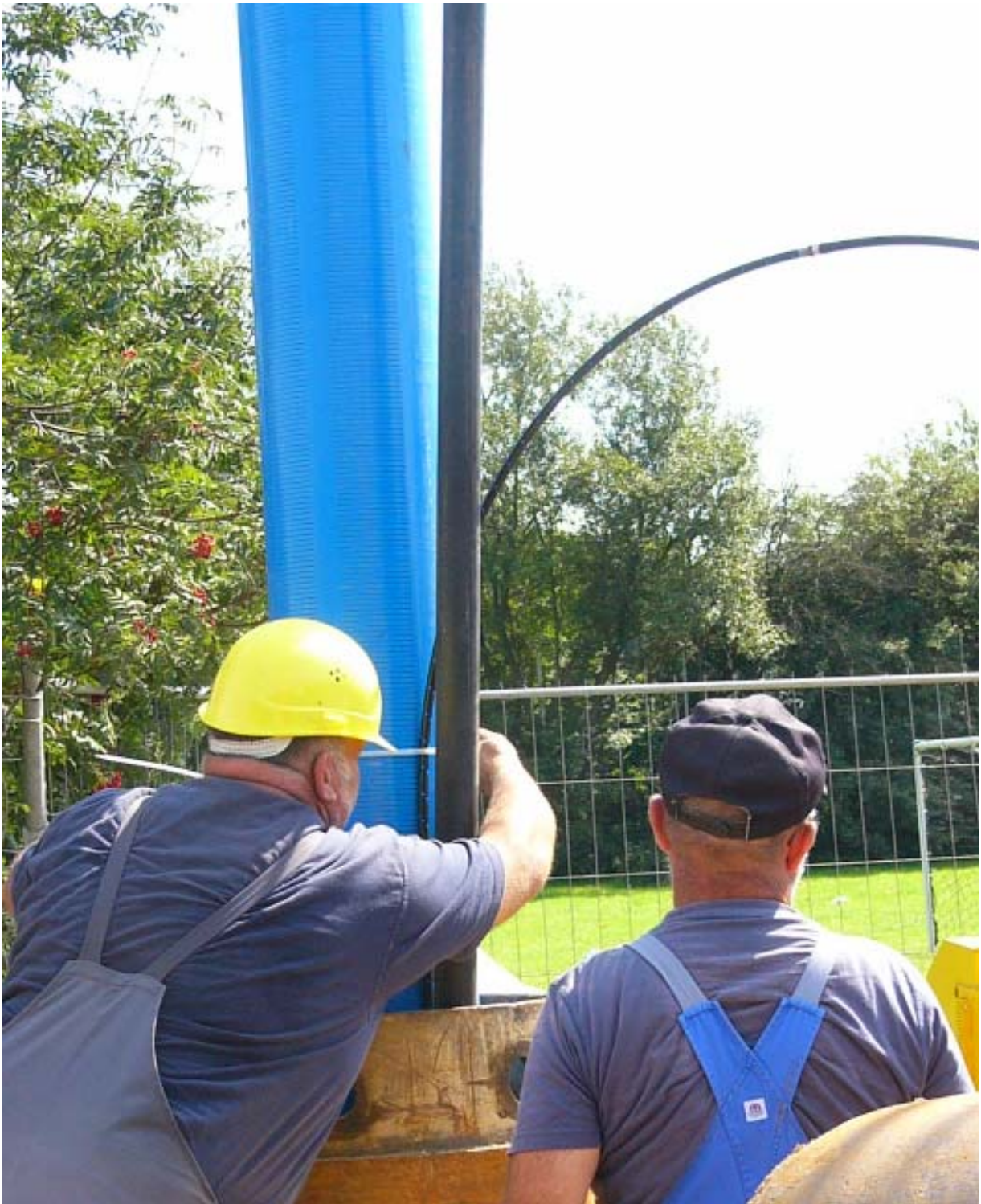
Installation of riser pipes of GASSYS and 2" piezometer (black) along pipe of remediation well (blue).
