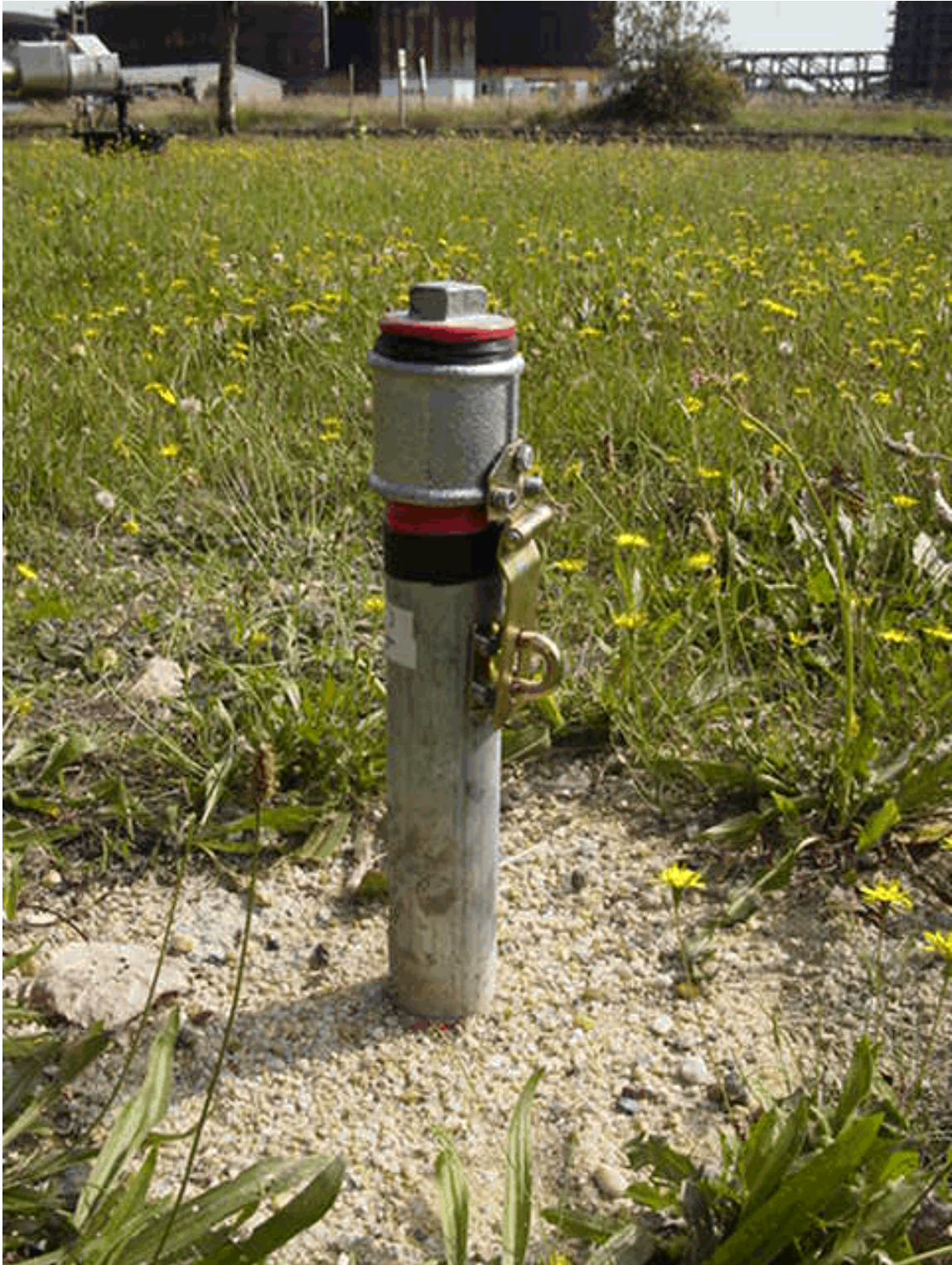
GASSYS installation above ground.
