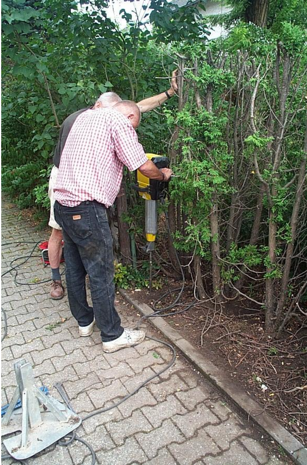
Drilling a small diameter hole with a hydraulic hammer. This drilling method can be used in tight spots. Other small diameter drilling systems could also have been used.
