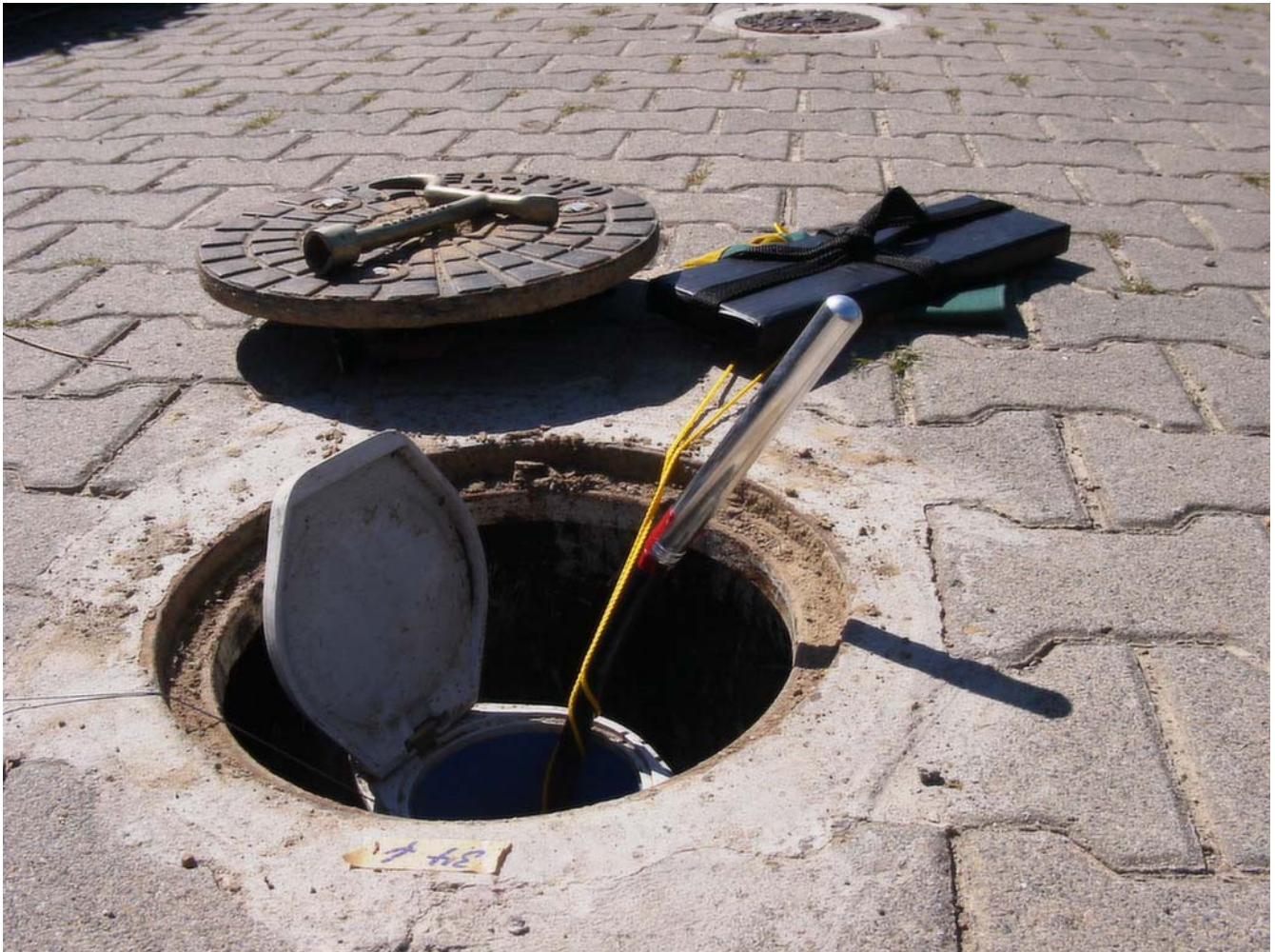
Access to installation below ground in a paved area at a plant site.
