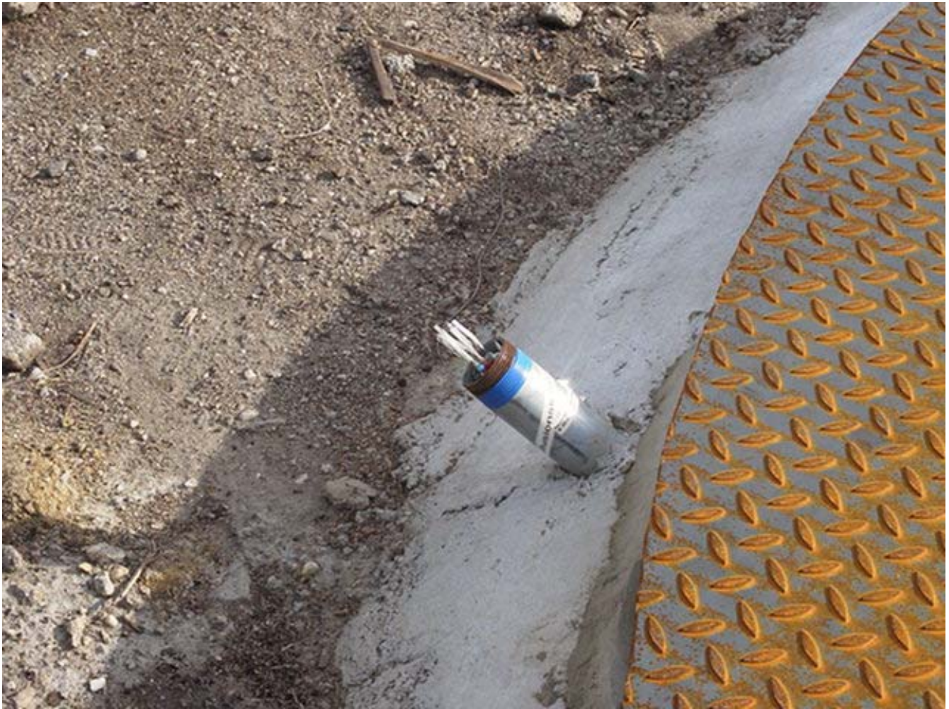
Oblique installation at a plant site.
