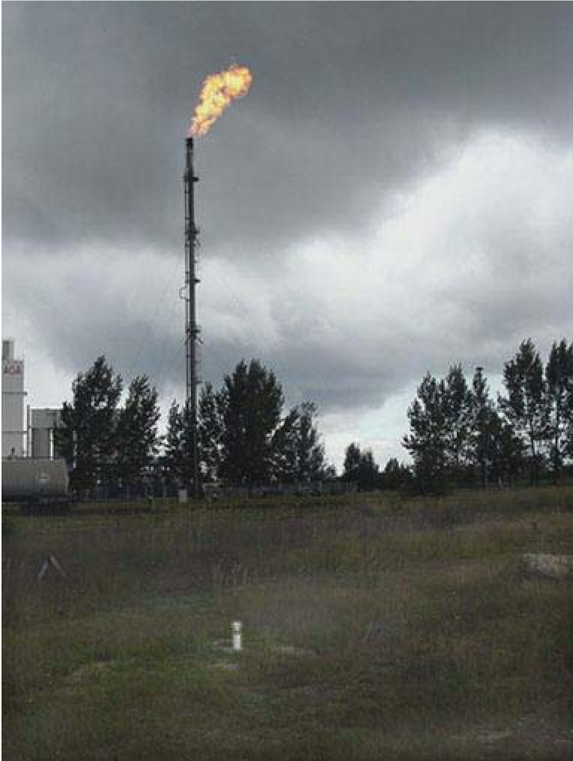
GASSYS installation above ground at a plant site.
