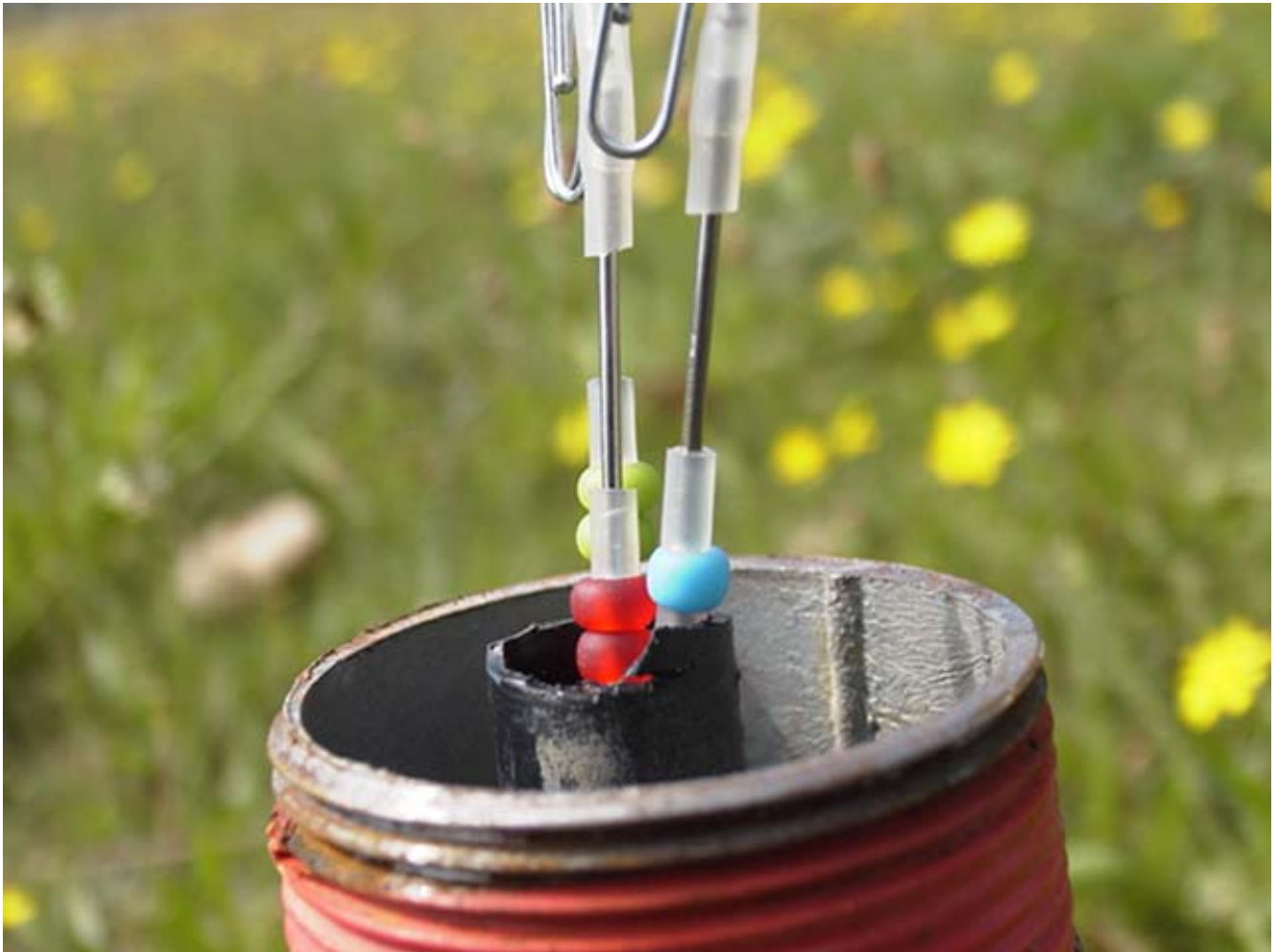
Access to GASSYS installation above ground.
