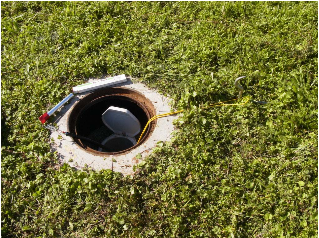
Access to GASSYS installation below ground in the field.
